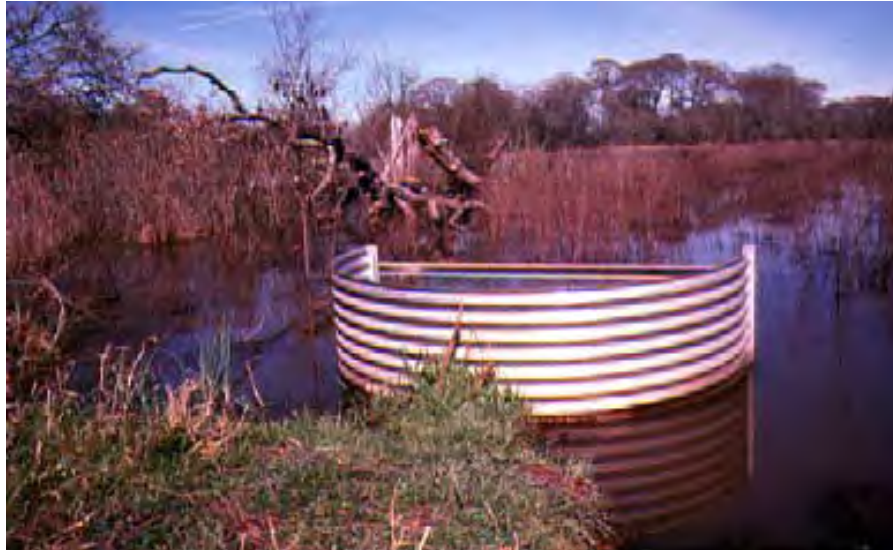
A flashboard riser box attaches to a pipe installed in a levee to create a shallow water wetland for wildlife.
